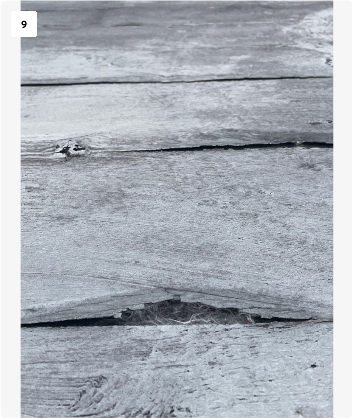
Cracking/damaged roof seams
