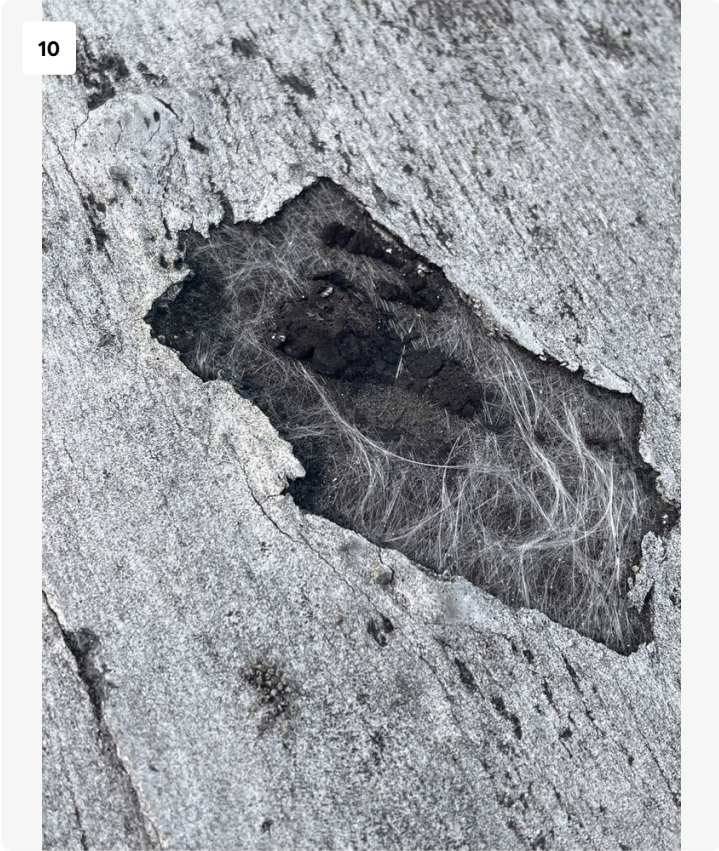
Asphalt smooth membrane showing damage, felt layers showing at seams and deteriorating coating
