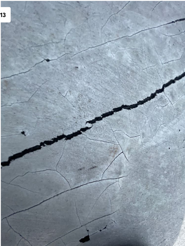
Cracking/damaged roof seams
