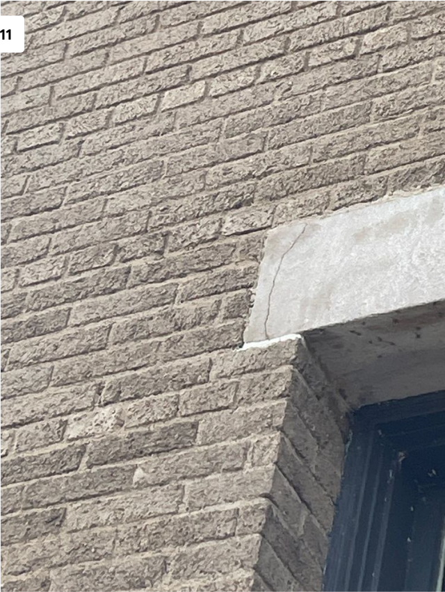
Damaged limestone header on first floor
