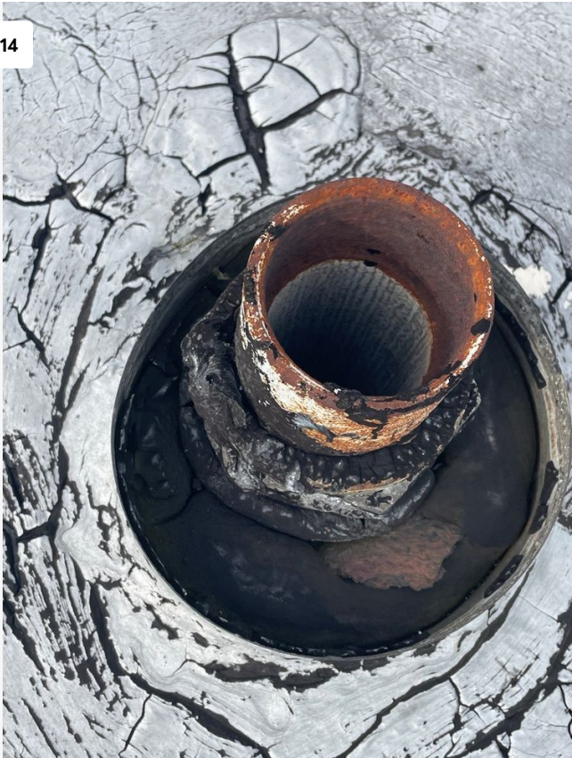
Failing pitch pocket needs new asphalt or 2 part pourable urethane.
