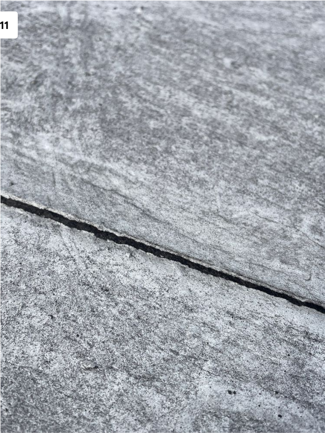
Cracking/damaged roof seams
