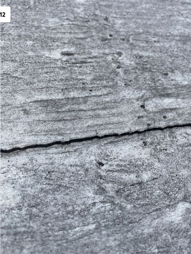
Cracking/damaged roof seams
