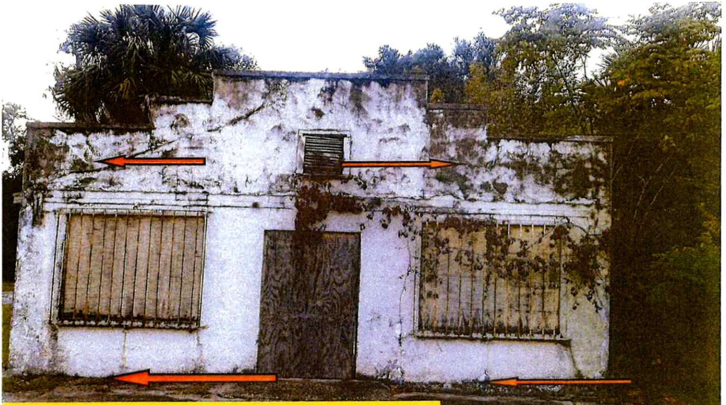
CASE #2024—184 709 N 12TH ST 1—A NOVEMBER 20,2024 DAVID GREEN Section 30-169 Mold and Mildew
