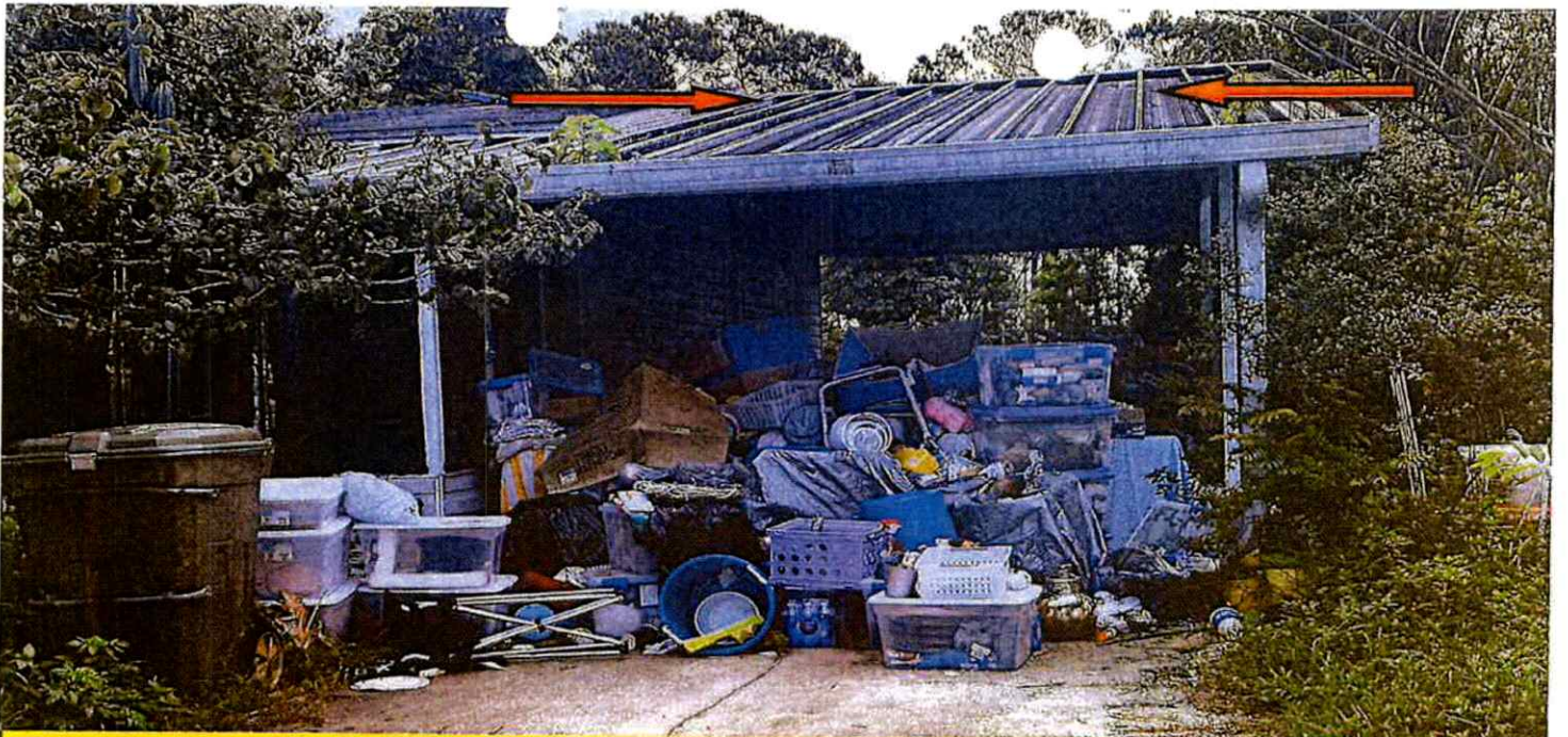
CASE #2025-025 105 VIKING ST 1A JULY 8, 2025 HAROLD BARTELLI PICTURE TAKEN FROM VIKING ST VIOLATION: SEC 30-169 MOLD AND MILDEW ON ROOF CARPORT
