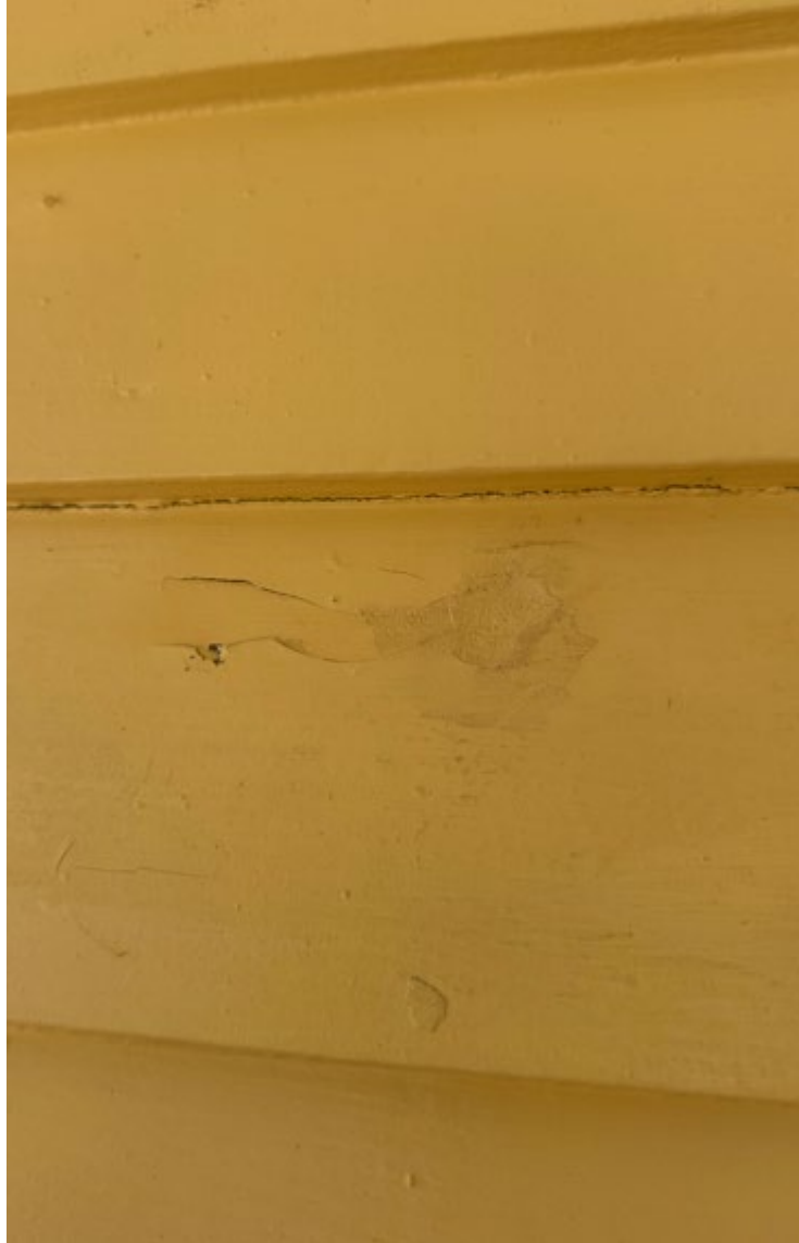
Figure 9: Current siding and paint to be repaired.
