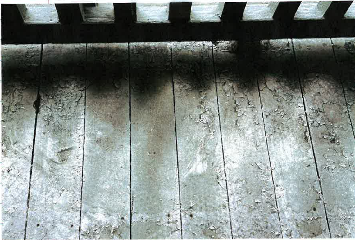
(17) FRONT PORCH (FLOOR)
