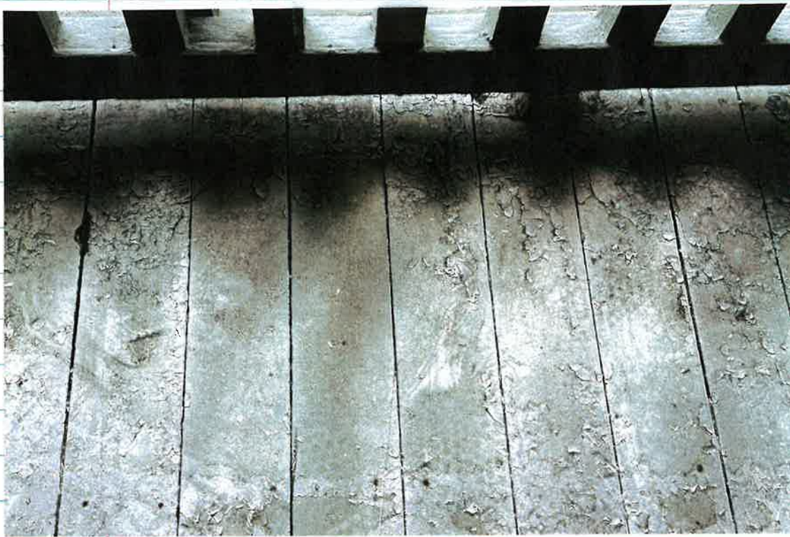
(17) FRONT PORCH (FLOOR)
