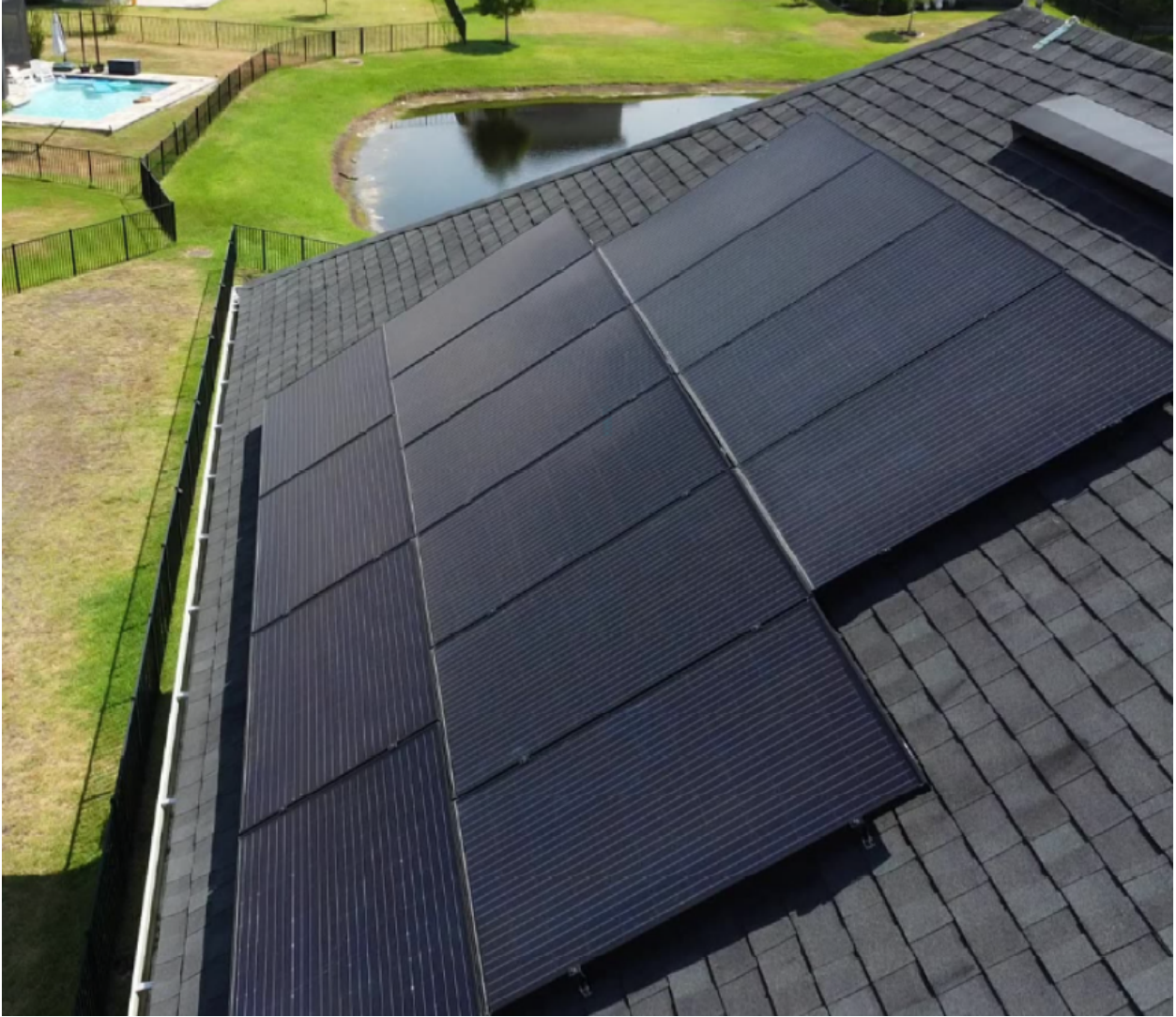
Figure 6: Bluenergy Solar Panels
