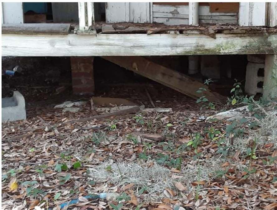
Rear Porch: Broken joist in contact with the ground; brick pier; block support without mortar and oriented with open cell horizontal; deteriorated and missing porch floor.
