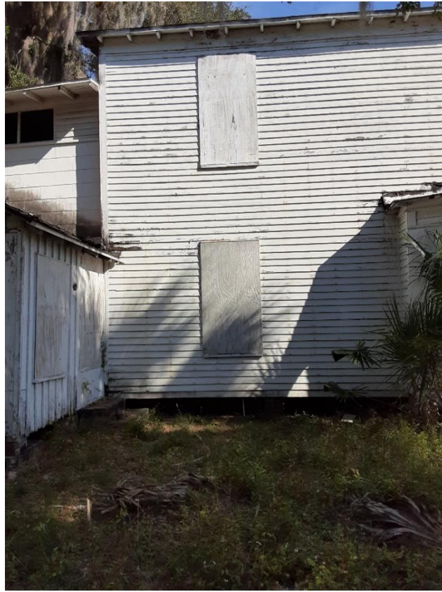
Left (West) Side View: Off grade construction; Relatively flat lot; Overgrown vegetation; Separation/Crack at roof intersection with side wall; Siding.
