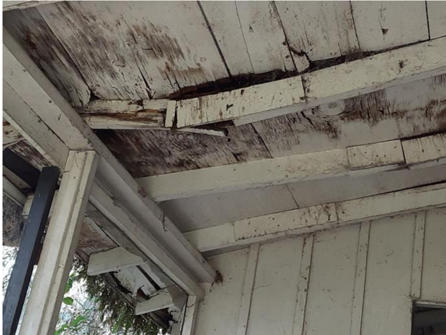
Rear Porch: Spliced and Broken Rafter; Deteriorated/broken soffit; Rotted outlookers (roof overhang supports).
