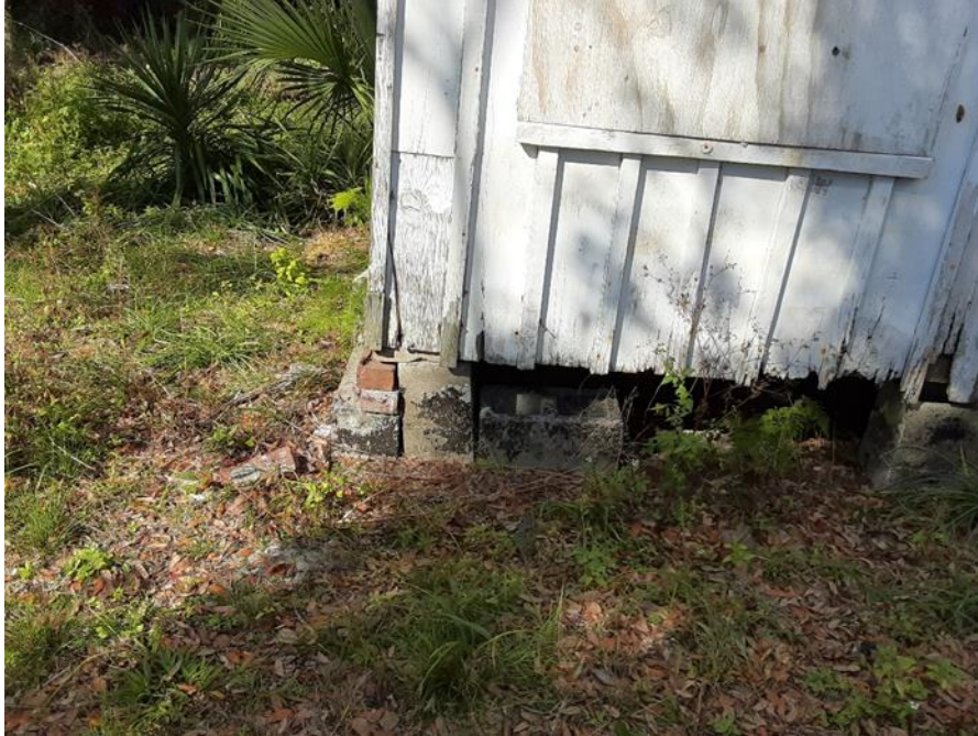
Pier: Leaning and Propped Concrete block
