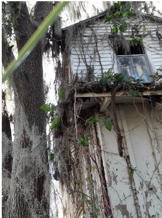
Rear and Right Side: Vegetation impacting structure; damaged siding; deteriorated roof edge and overhang; broken window.
