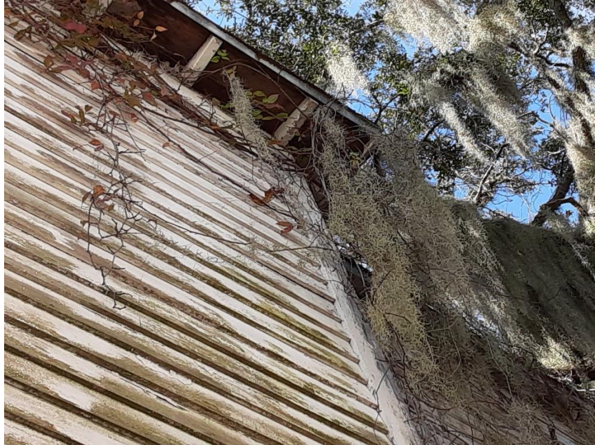
Right (East) Wall and Roof Overhang: Mildewed siding and growing vegetation.
