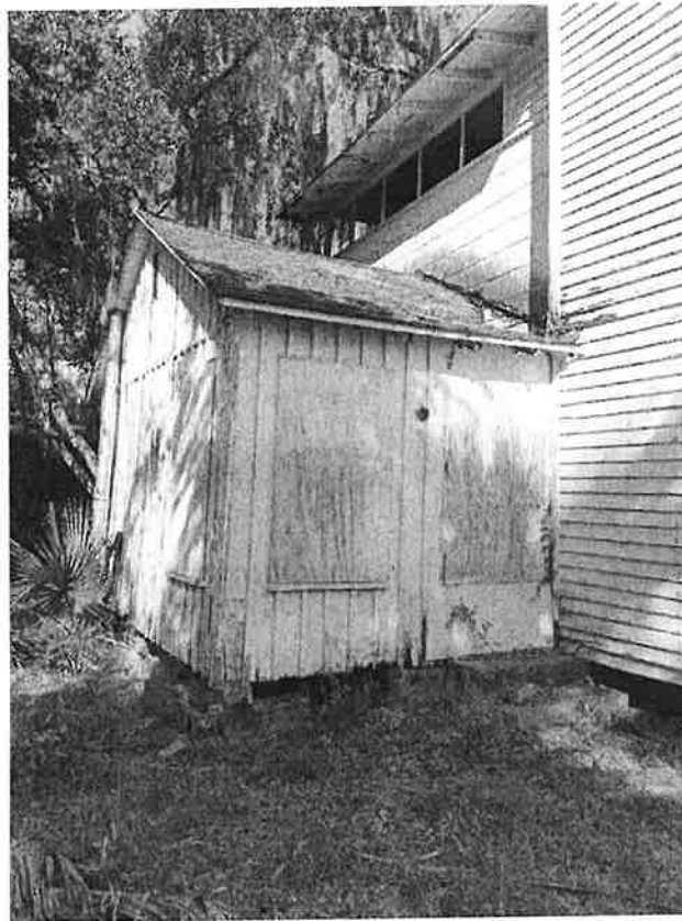
Left-Rear (North-West) View of Possible Addition: Roof Separation and patching. Deterioration of siding at bottom; Leaning pier with nearby loose blocks.
