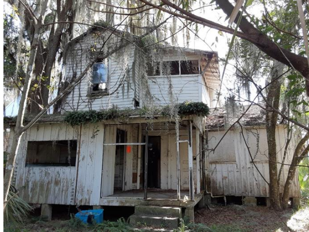
Rear (North) View: Overgrown vegetation close to structure and in contact with roof.
