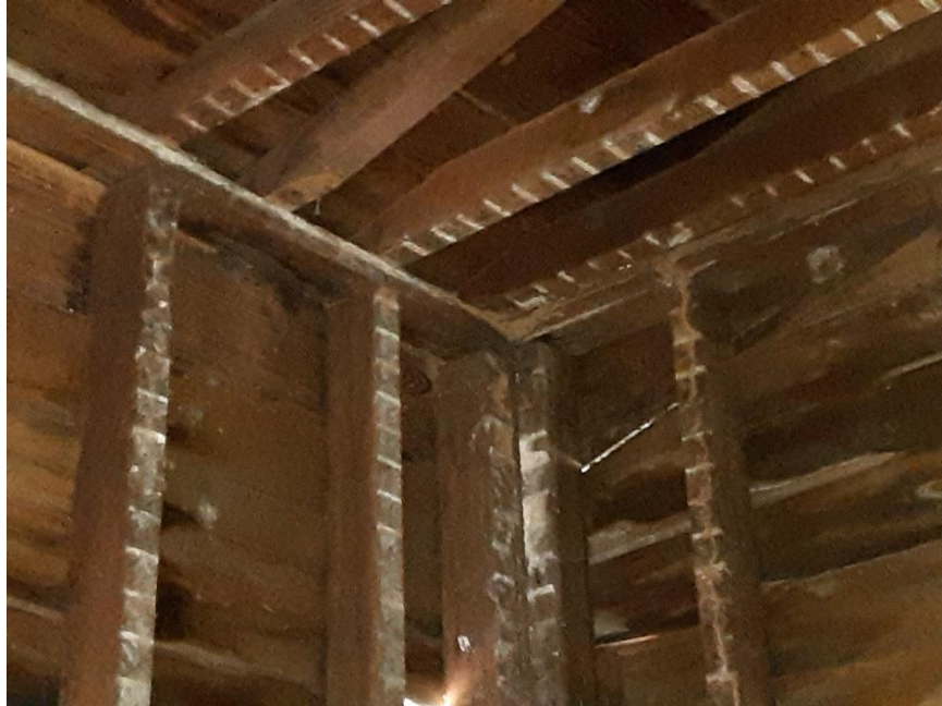
Second Floor Roof and Wall Corner Framing: The picture does not show a double top plate; No hurricane clips or other metal connectors are present.
