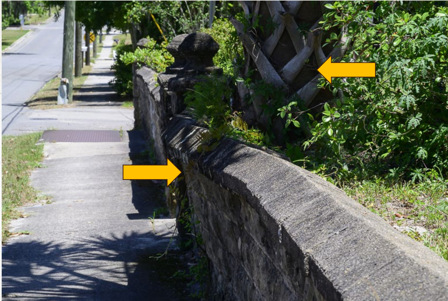
Vegetation has pushed up against the wall causing further damage.
