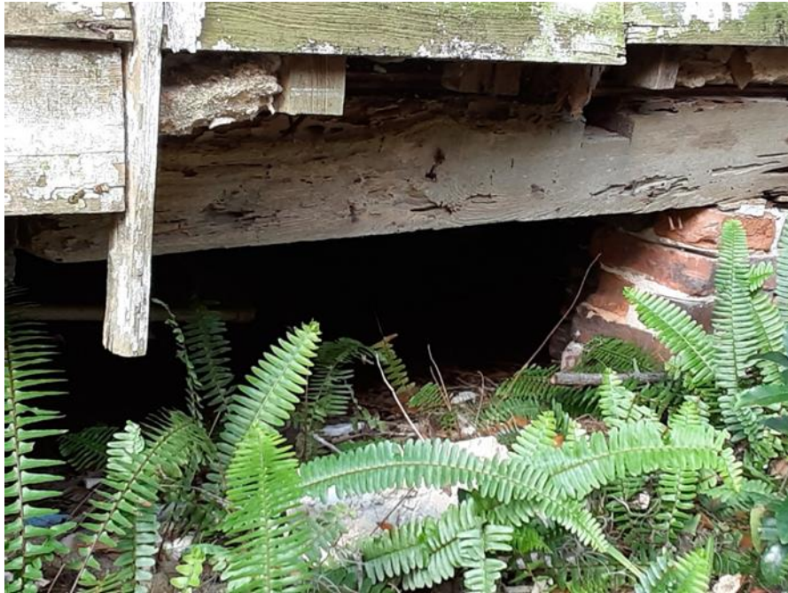
Right (East) Sill Beam: Deteriorated/Rotted/WDO damaged sill beam.
