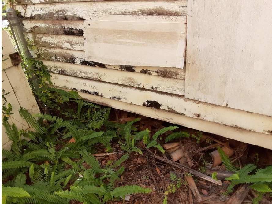
Right-Front (South-East) Lower Corner: Nearby vegetation; Mildewed Siding.
