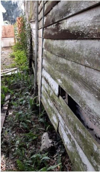
Right (East) Wall Siding: Damaged and Missing siding.
