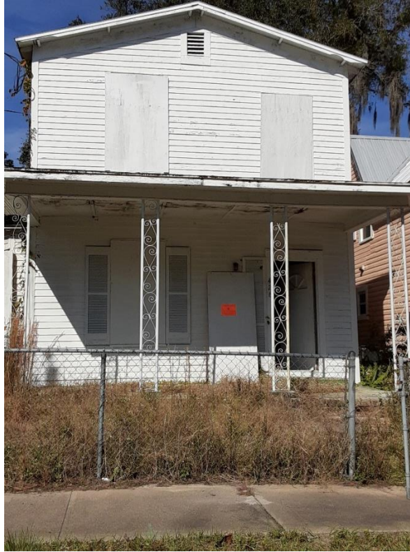
Front (South) View: Showing stained/damaged/deteriorated wood soffit (ceiling) on the front porch.
