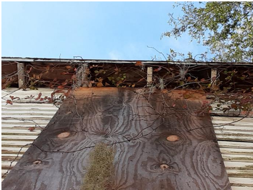
Right (East) View: vegetation growing on wall and along roof overhang area.
