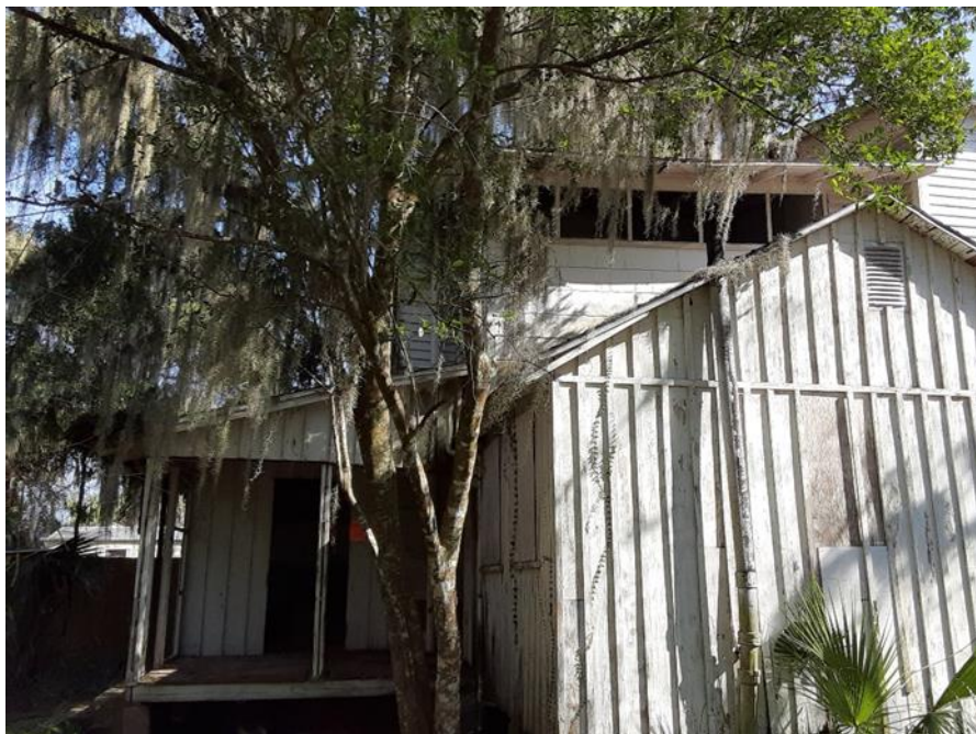
Rear Porch viewed from Left (west) side: The rear porch appears to be distorted (as if leaning toward the house). Perhaps, the orientation of the camera contributes to this slant. However, the rear porch is in very bad condition and needs to be demolished. A tree and other vegetation are growing very close to the structure.
