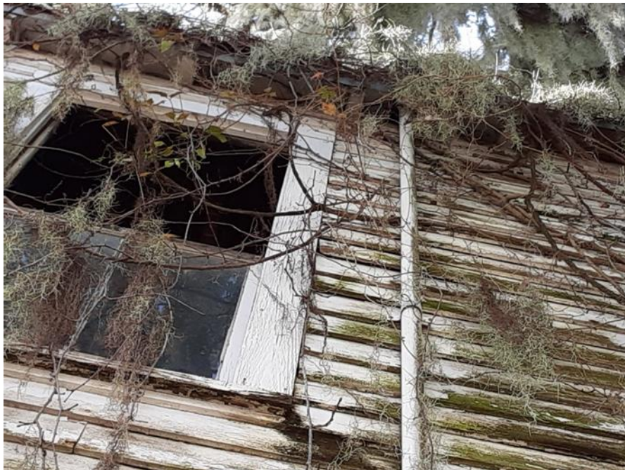
Right (East) Wall and Roof Overhang: Mildewed siding, vegetation, broken window and downspout.
