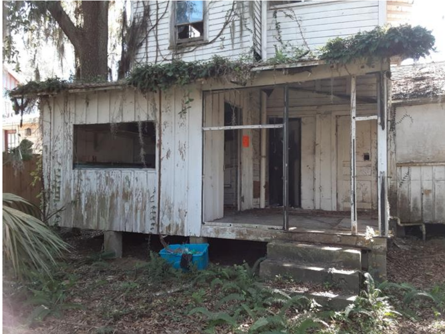
Rear (North) View: Rear porch and side room with vegetation on the roof and walls; crack in rear step.
