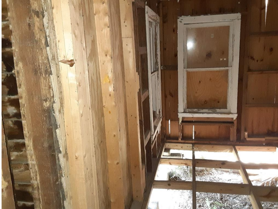
Left Rear (West-North) Room: Incomplete Wall and Floor Repair
