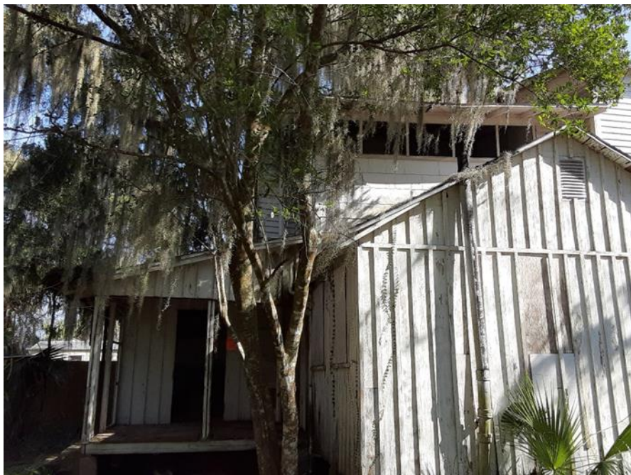
Rear Porch viewed from Left (west) side: The rear porch appears to be distorted (as if leaning toward the house). Perhaps, the orientation of the camera contributes to this slant. However, the rear porch is in very bad condition and needs to be demolished. A tree and other vegetation is growing very close to the structure.
