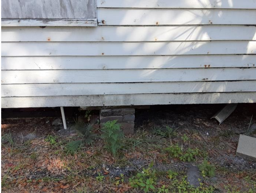
Pier: The photograph appears to show with added wood and loose blocks at top of brick pier
