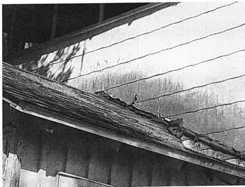
Left-Rear (North-West) View of Possible Addition: Roof Separation and patching.
