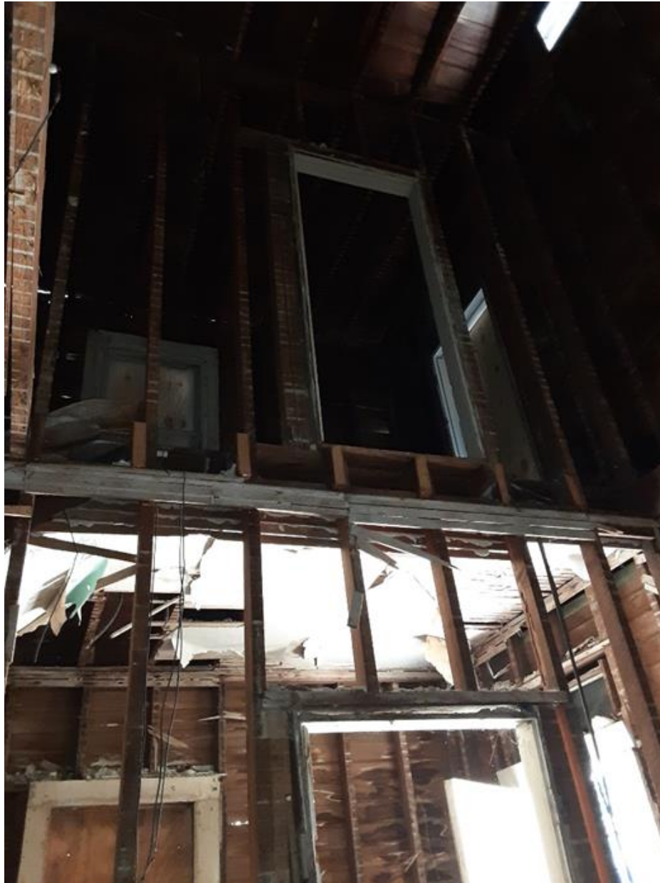
Interior Wall Framing: View from Down Stairs Looking to Upstairs; studs in good condition, cut and removed ceiling/floor joists supporting second floor.
