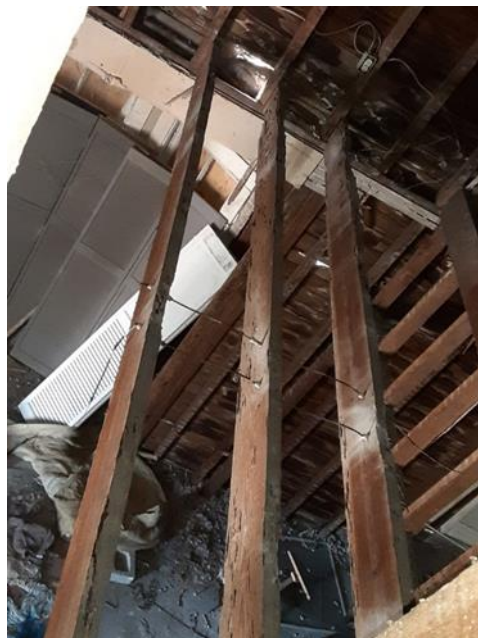
Ceiling/Floor Joists Supporting Second Floor: Deteriorated members; some missing.
