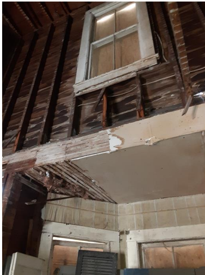
Exterior Wall: Walls and Window framing: very good condition of the studs and some other structural members; damage shown may have resulted from demolition activities.
