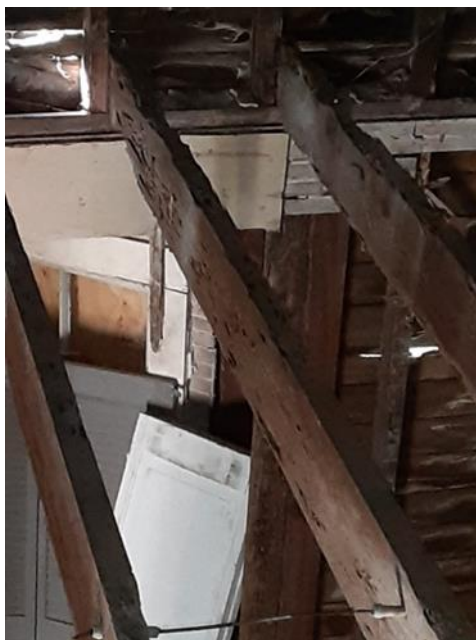
Rotted/deteriorated ceiling/floor joist (front (south) room area). Some of the joist had been removed.
