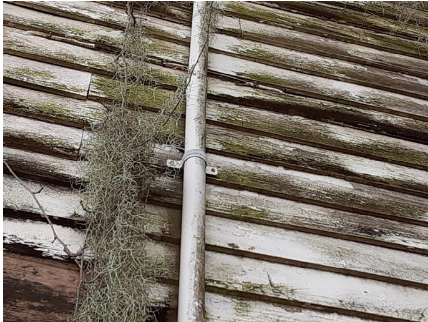
Right (East) Side Wall: Downspout, damaged and mildewed siding.
