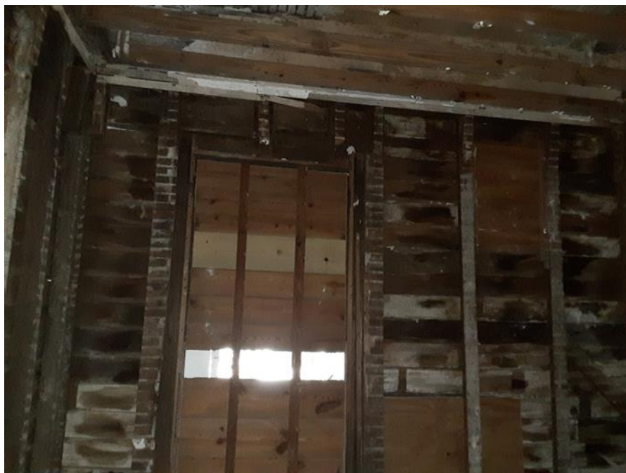
Exterior Wall Right (East) Side: Missing Siding and Discolored Siding.
