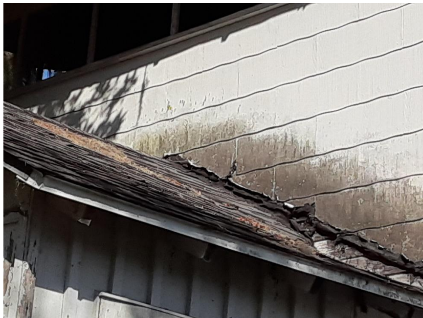
Left-Rear (North-West) View of Possible Addition: Roof Separation and patching.
