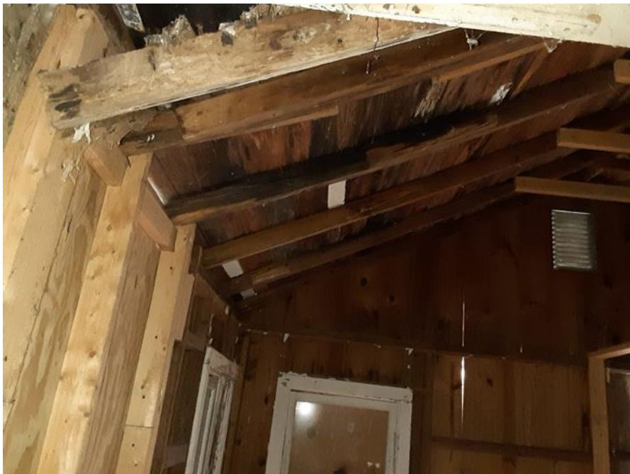
Left Rear (West-North) Room: New collar ties and wall construction; damaged and sliced rafters; water stains and holes in roof decking.
