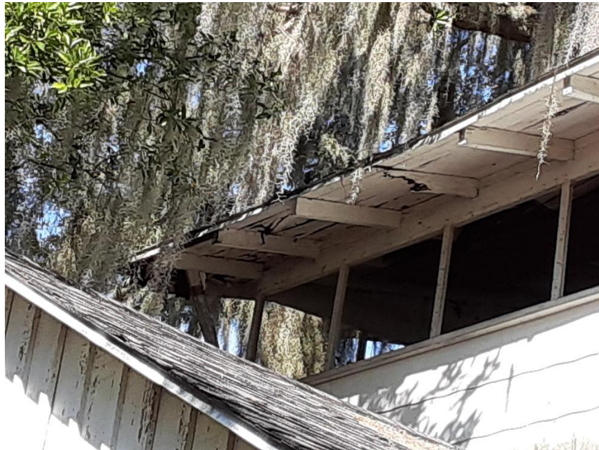
Second floor Roof Overhang: Damaged and deteriorated roof decking and outlookers
