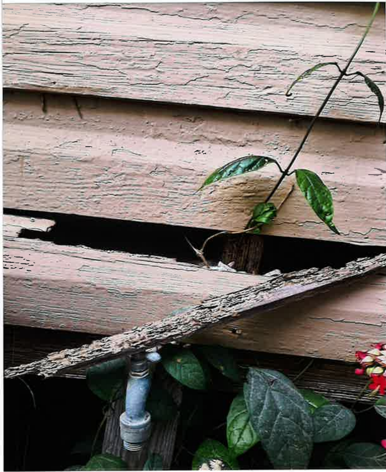
EXTERIOR ROT + WEATHERING
