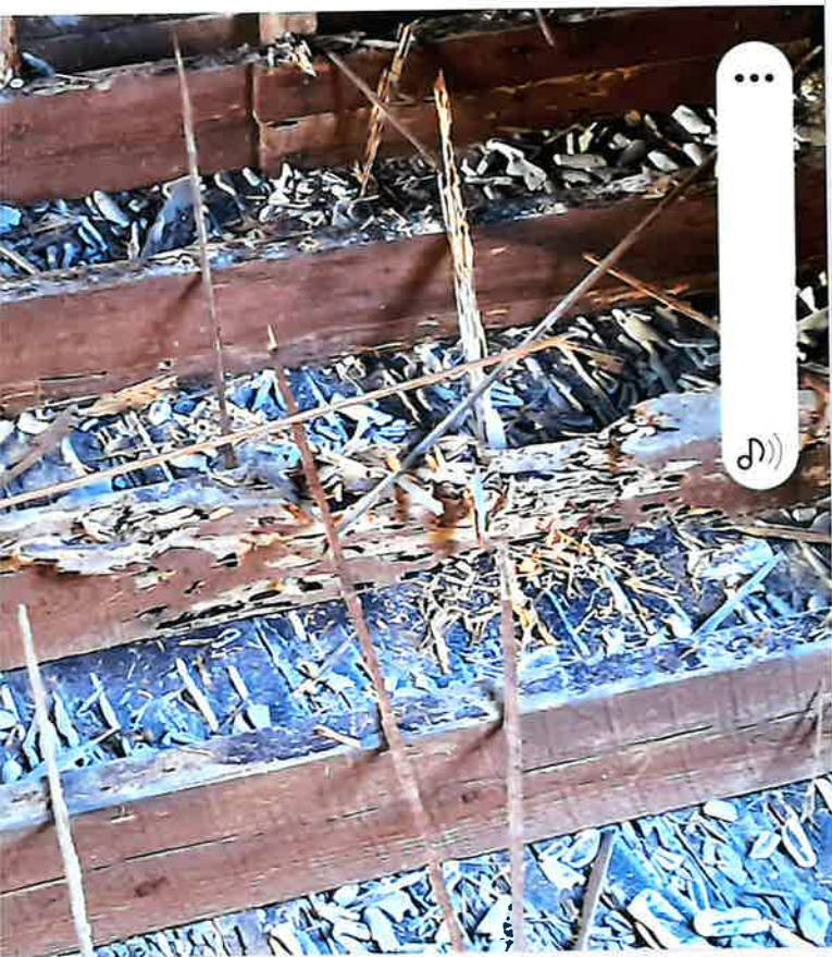
2 ND STORY FLOOR JOIST ROT AND TERMITE DAMAGE
