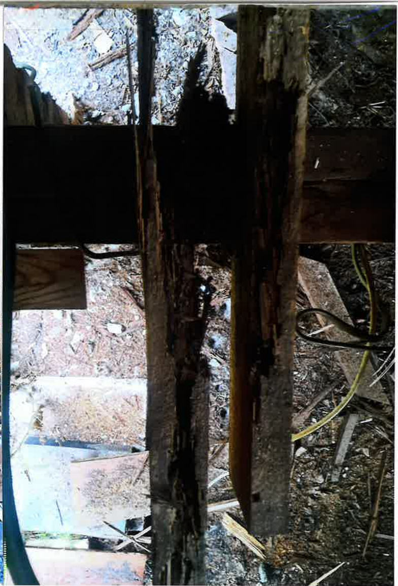
1 ST FLOOR JOIST ROT AND TERMITE DAMAGE
