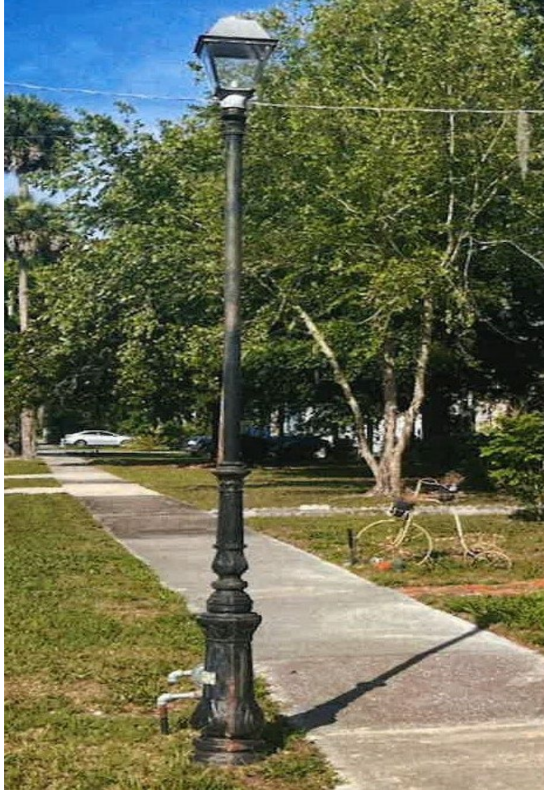
Figure 4: SHD Existing lamp posts.
