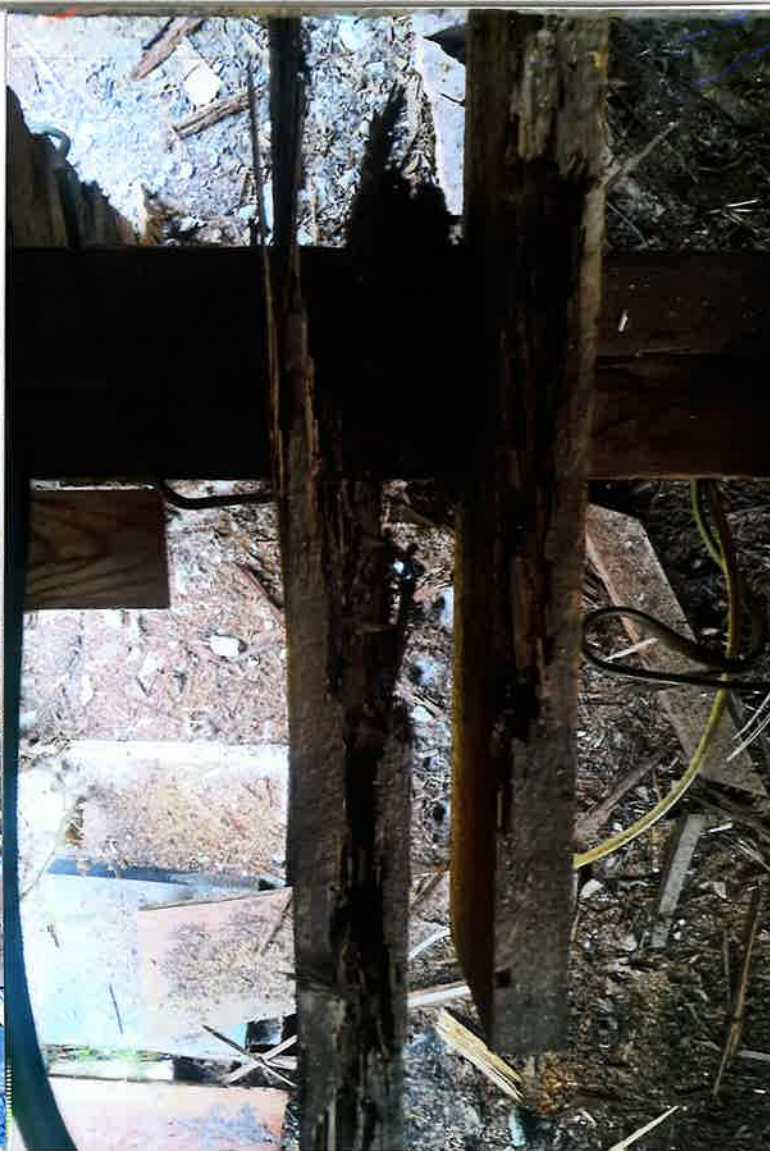
1 ST FLOOR JOIST ROT AND TERMITE DAMAGE
