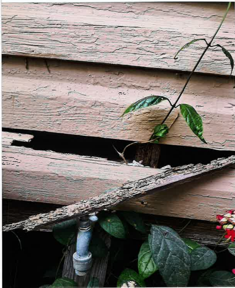
EXTERIOR ROT + WEATHERING
