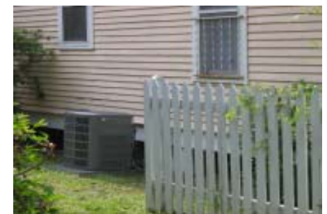
Mechanical equipment should be screened from view.
