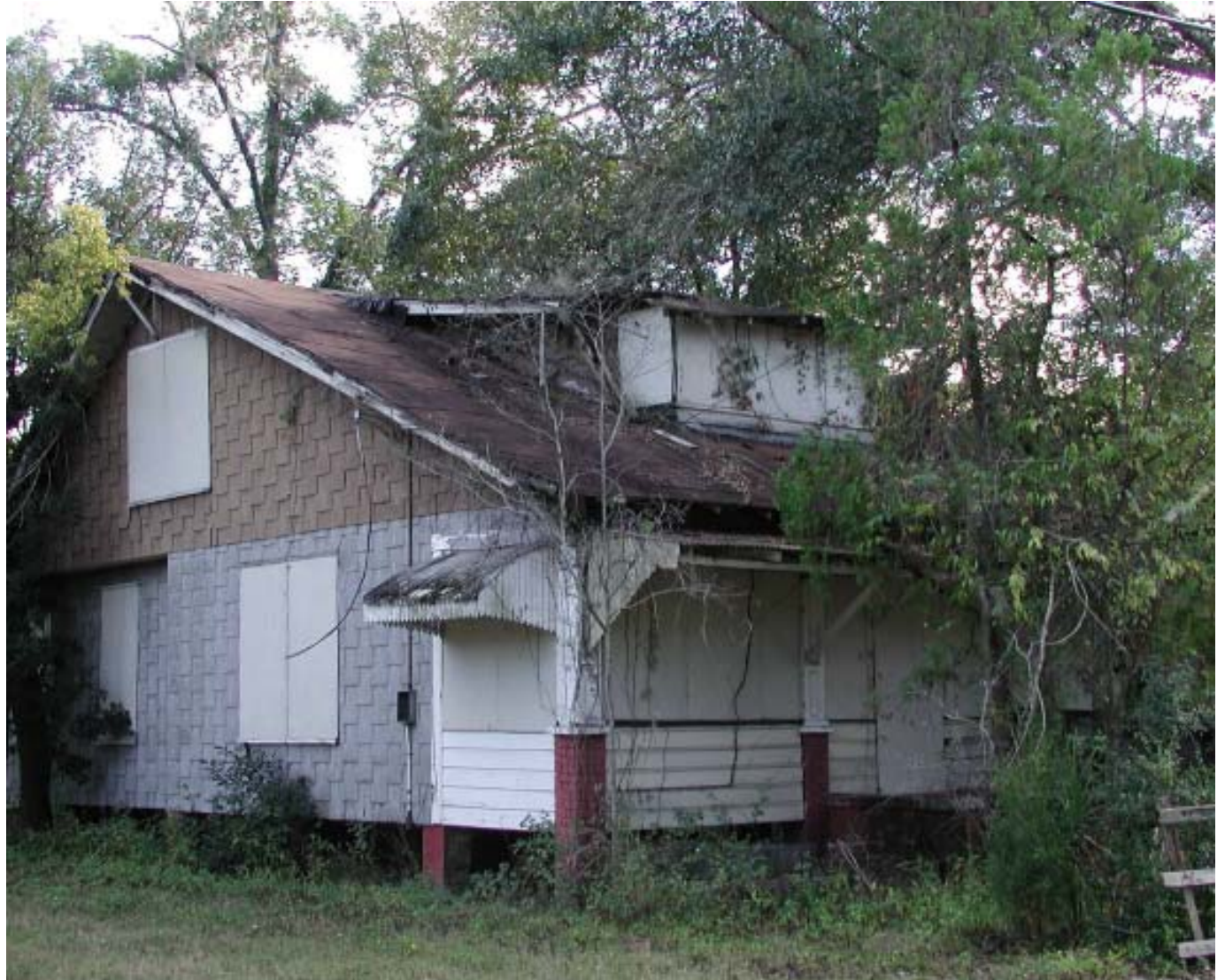
Many historic and contributing structures have faced demolition due to fire damage and deterioration.
