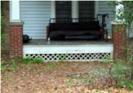
Lattice infill at pier foundation in University Heights North Historic District.
