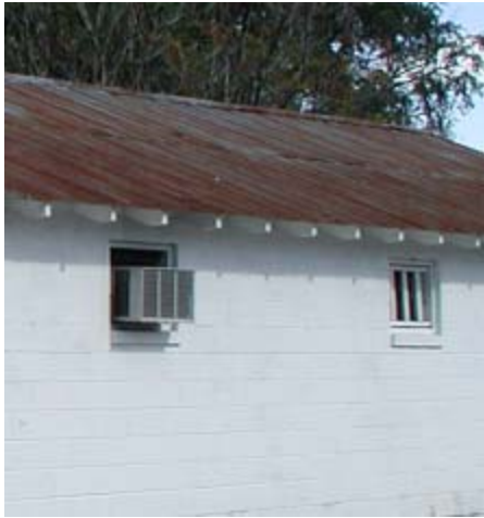
Avoid radically changing the appearance of a historic building with mechanical units.
